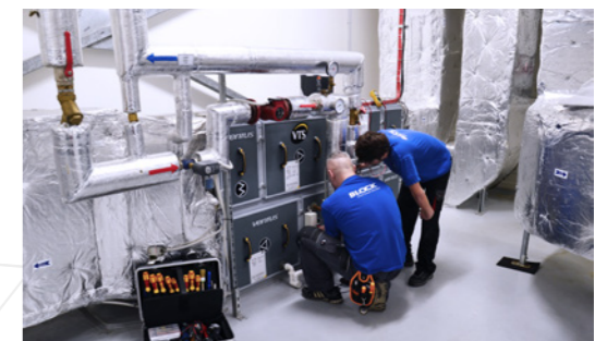
Wiring, Measurement and regulation
