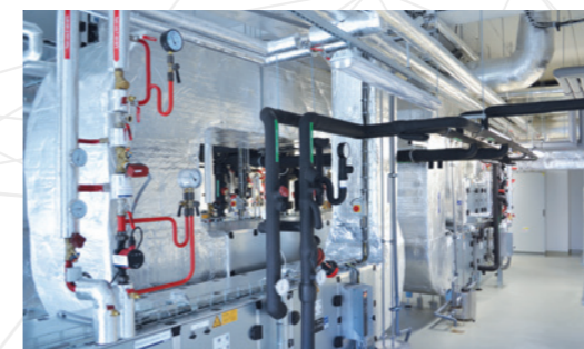
HVAC (heating, air conditioning, cooling)
